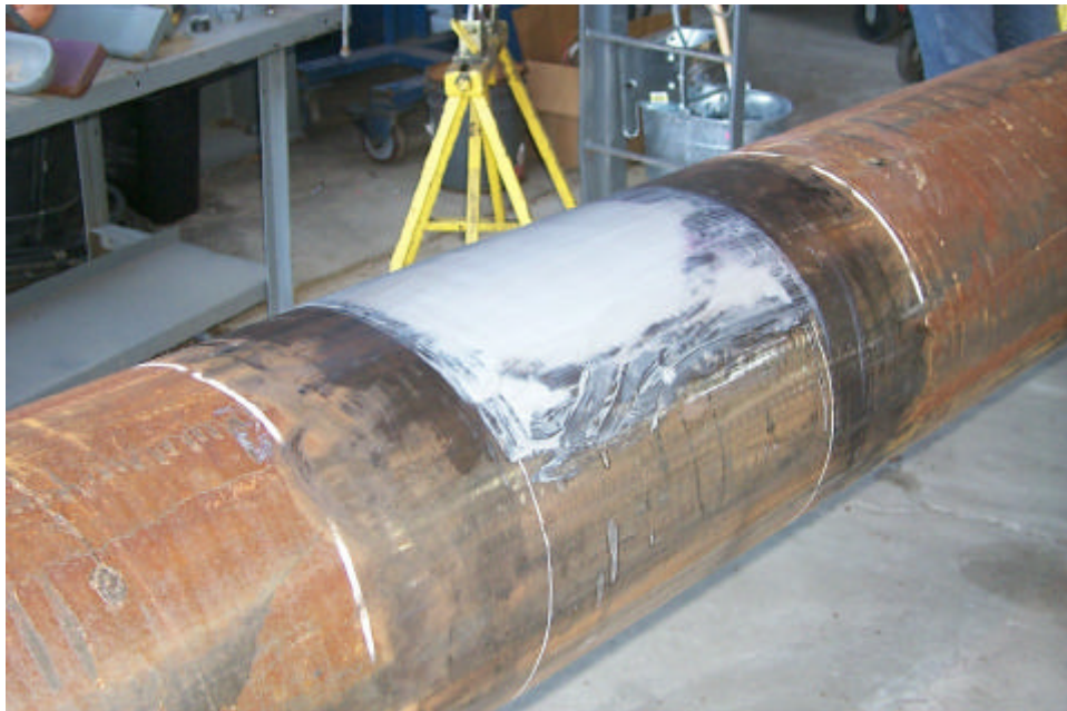
Figure 4 Filler material applied in dented region
